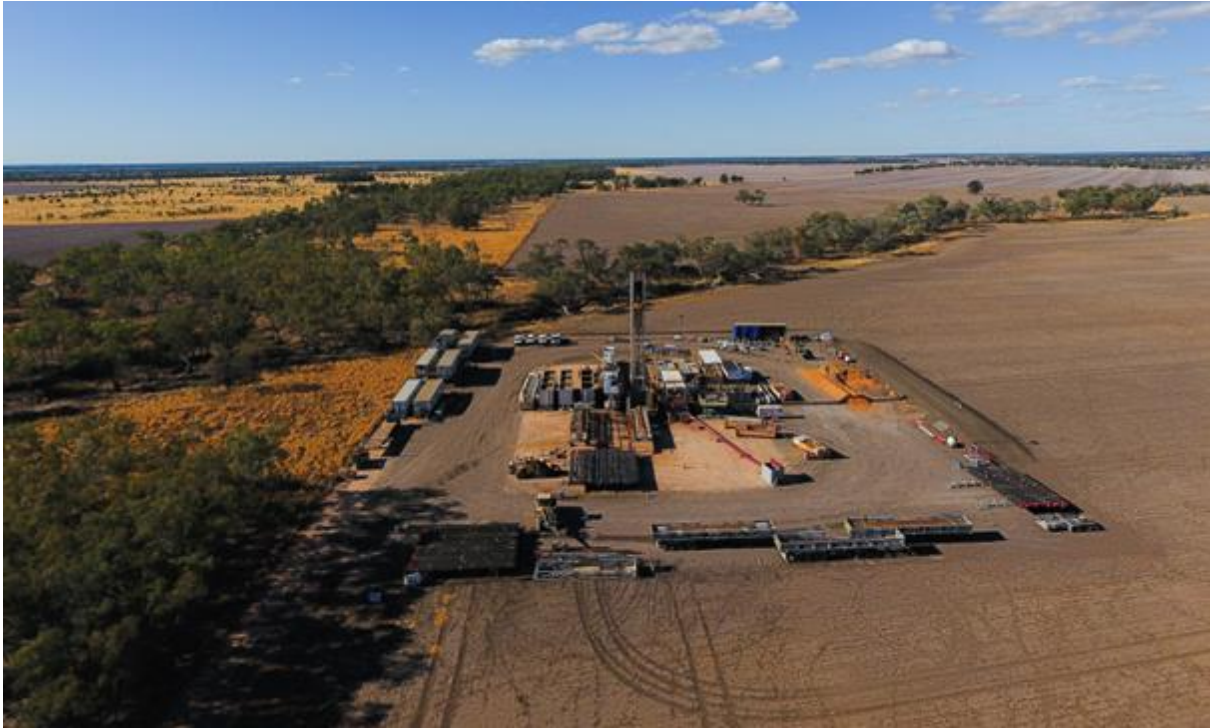
Plate 4-1: Example of an onshore drilling rig 13
