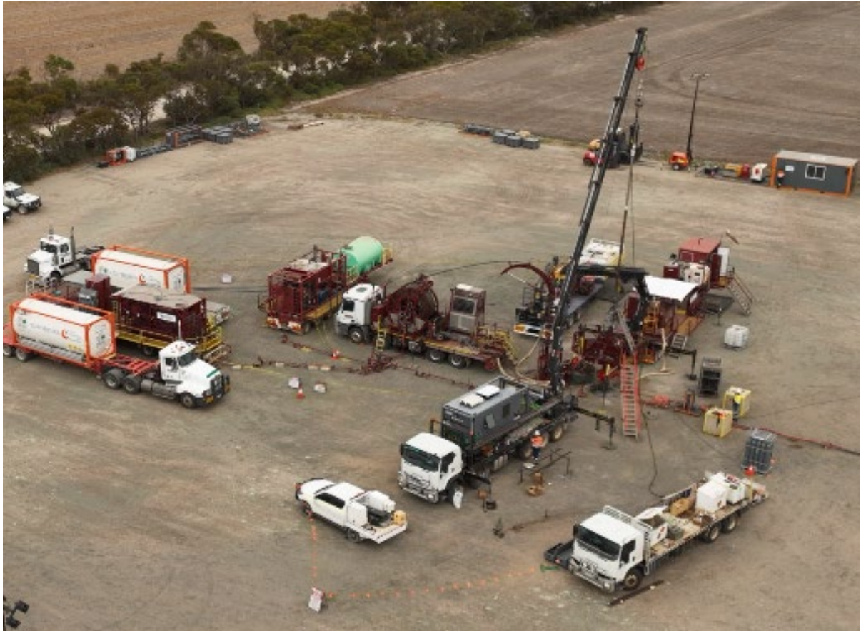
Figure 3 – Exploration Well Testing Equipment on Site at Ramsay 2
